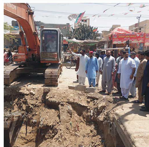
Chairman Sohrahb Goth Town Lala Abdul Rahim is inspecting the steps taken To restore the sewerage system in Ahsanabad.
